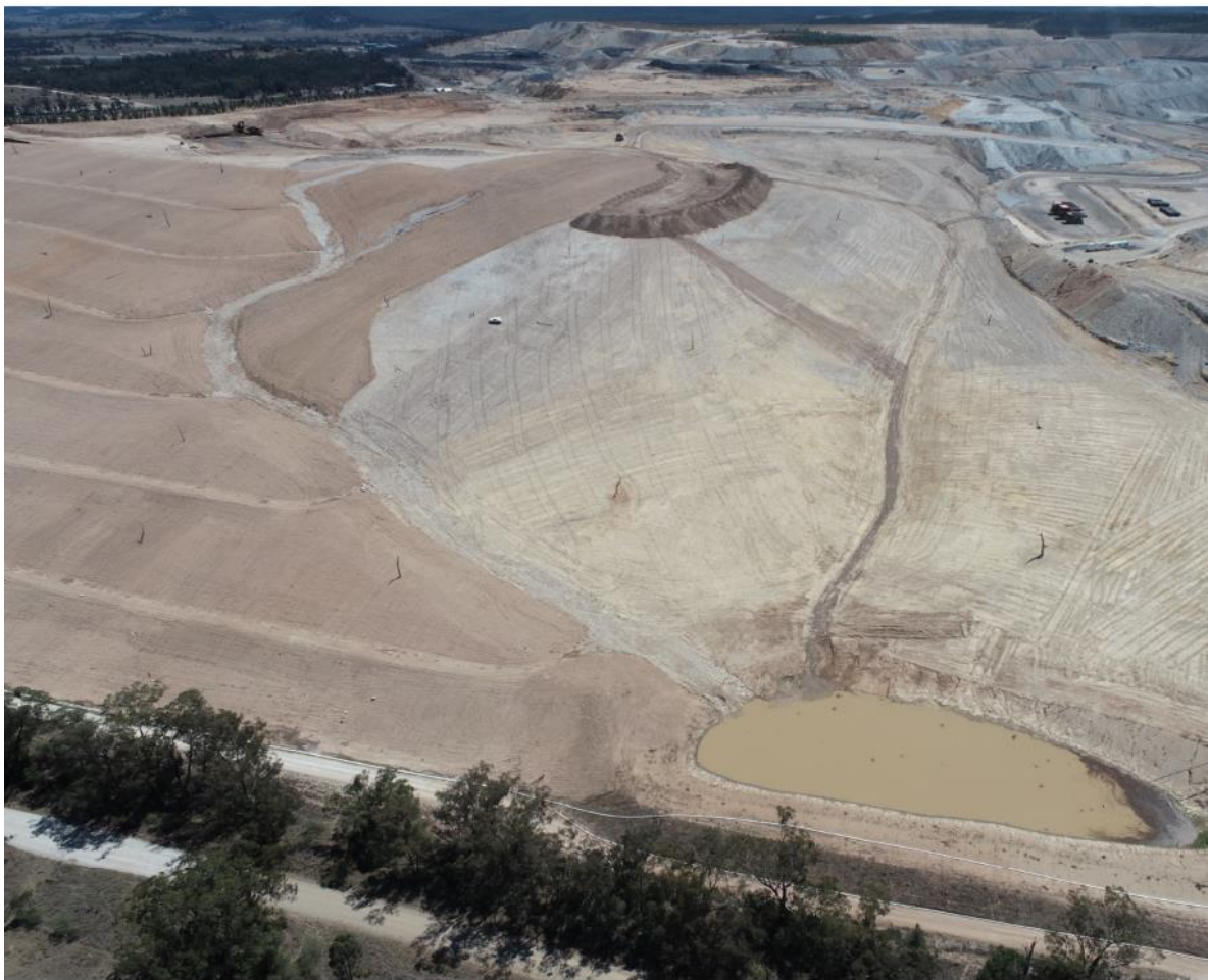
Photo taken in October 2023 displaying topsoil spreading activities on the Southern Emplacement Area
