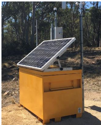
Portable and real-time dust monitor installed at TCM in November 2018
